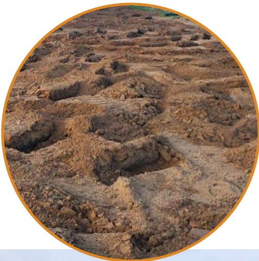
Example of Uneven Scarification
