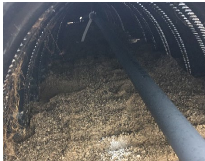
- SBT with pressurized distribution piping in a leaching chamber
